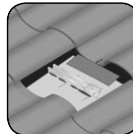
Step 7: Install subflashing and seal as needed if double flash is desired.
